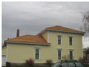
The Adler House Museum has a new roof thanks to grants from the Leo Adler Foundation
